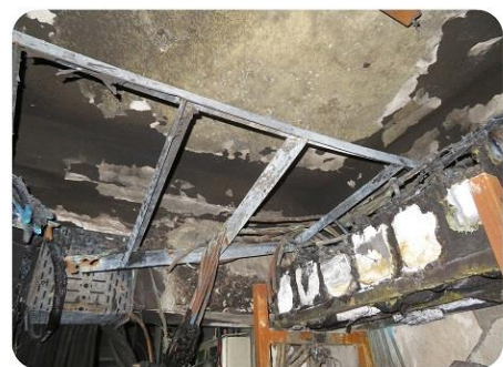
Figure 2: Thermal runaway destroys battery racks at a data centre used by a mobile phone operator in DRC - CEERISK 2017
